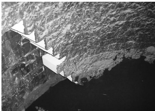
图 4 下部槽第一次更换环流管时的槽壁刚玉-尖晶石材料 Fig.4 Corundum-spinel materials used in lower vessel walls
